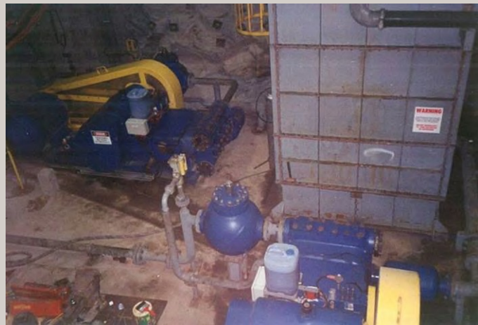
Underground Pump Station at KCGM's Chaffers Shaft
